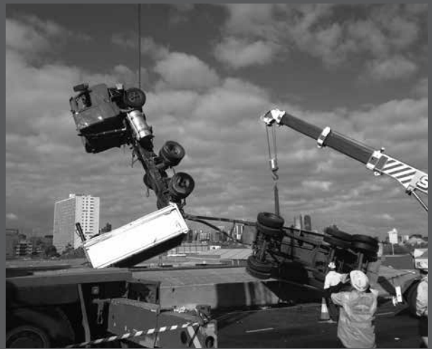
Crews work to remove the overhanging truck from the CityLink onramp.
