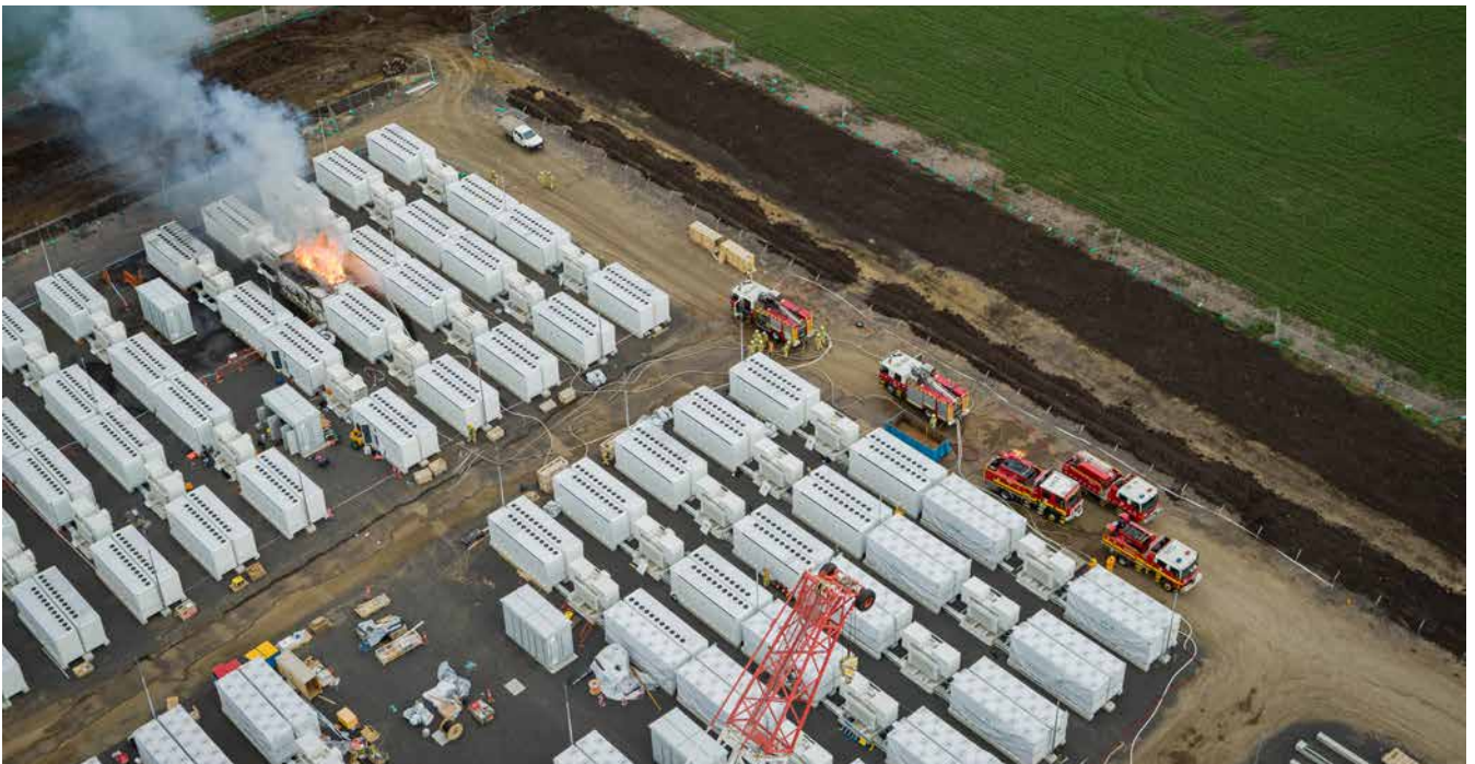
Moorabool battery fire 30 July 2021
